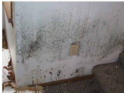
Aspergillus found behind wall baseboards
