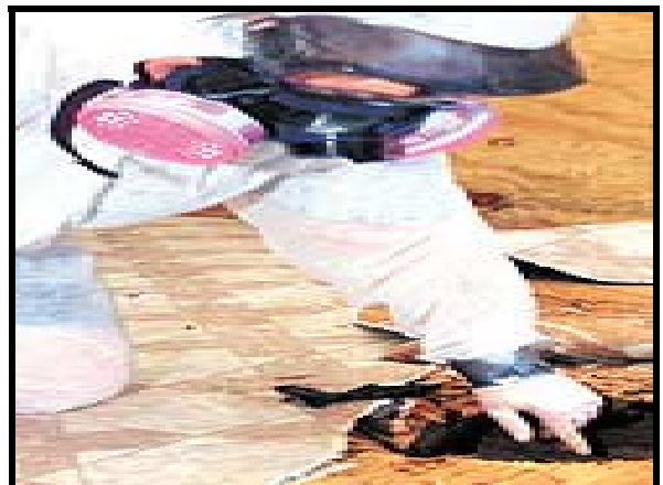
Figure 1: Mold remediation in a Kitchen
